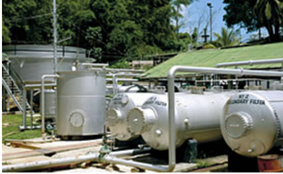
Domestic Water Treatment facility at Pointe-a-Pierre. This is a crucial part of the utilities infrastructure
